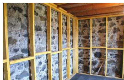
Installing an internal frame, infilled with insulation and a plasterboard finish is relatively simple and inexpensive. In this example, the frame is set apart from the wall to avoid moisture in the stonework affecting the new works.
