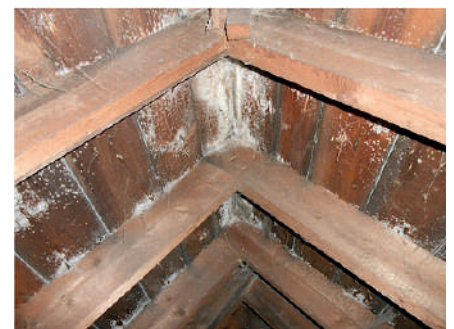
A consequence of warm, moist air entering the loft area but not being adequately ventilated away, hence the importance of ventilation at the eaves
