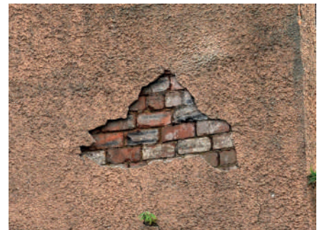
Render fallen from a brick wall. It is likely that adjacent render is 'boss' (loose) and repair is urgently needed
