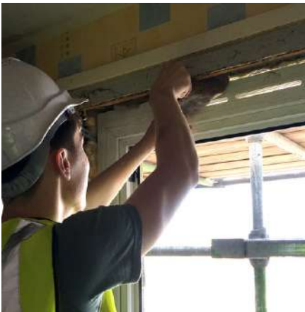
Expanding foam tends to become rigid and brittle leading to gaps through which air can travel. In this project sheepwool is being stuffed tightly into the gap. Sheepwool is preferable because it remains flexible.
