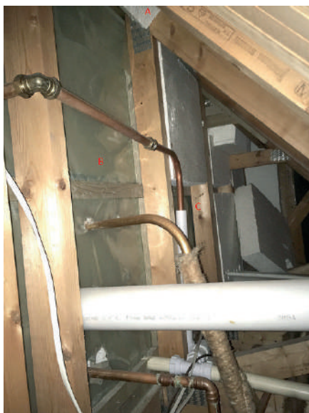
This shows the upstairs wall of the house shown on page 90. The polystyrene insulation has been removed to install pipes and nothing replaced, meaning that in effect, there is only plasterboard between the bedrooms and the outside air. In addition, the hot water pipes are uninsulated. Unfortunately, there's a lot of fiddly insulating and airtightness work to be done here.
