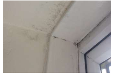
Example of mould / damage due to cold air behind plaster board or window reveal
