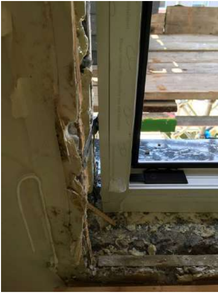
Brand new windows installed but note the gap around the frame which is normally sealed with expanding foam
