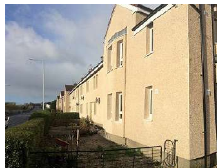
In this retrofit project, some of the decorative details of these houses have been lost through EWI. If we want to preserve the identity and enjoyment of places across Scotland then we will have to treat social housing like this with more of the care and attention typically spent on ‘conservation’ projects
