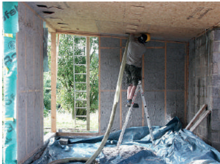
A timber framed 'breathing wall' under construction with hygroscopic recycled cellulose insulation being pumped into ceiling voids and already installed into the walls.
