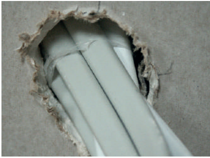
Cables protruding through plasterboard where no service void has been provided meaning the vapour barrier here has been breached
