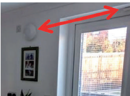
Extract fans placed near trickle vents will short circuit, meaning the rest of the room, and other rooms, can be under-ventilated
