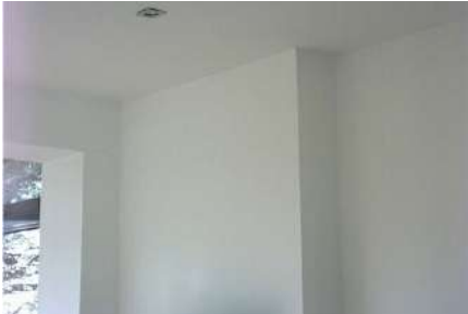
A clear example of thermal bypass. Cold air from the junction with a new conservatory is getting behind the plasterboard in the kitchen area and cooling the wall.
