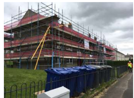
The costs of scaffolding are high, so if it is needed for one works package (e.g. window replacement) it makes sense to take the opportunity, as Renfrewshire Council did here, to also externally insulate and renew the roof finish
