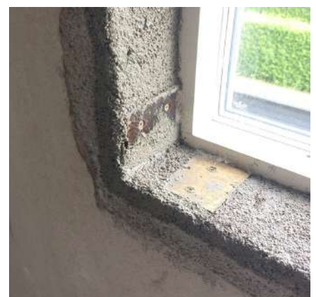
In this example, the reveal has been insulated with a natural, vapour permeable insulating plaster to counteract the poor performance of the thinner walls, and to complement the new windows
