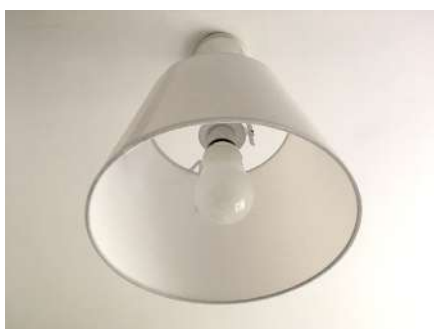
LED bulb in a standard bayonet light fitting. It looks like a traditional incandescent bulb but is far more efficient—this 15W bulb is roughly equivalent to an old 60W or 100W bulb. Note a white and simple shade, which does not obscure any of the light to the area directly beneath.
