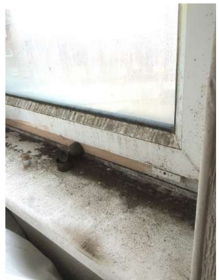
The trickle vent in this bedroom window was kept closed, as was the door, meaning there was not enough fresh air to clear the moisture in the air, leading to condensation and mould on the coldest available surface: the window frame and reveals
