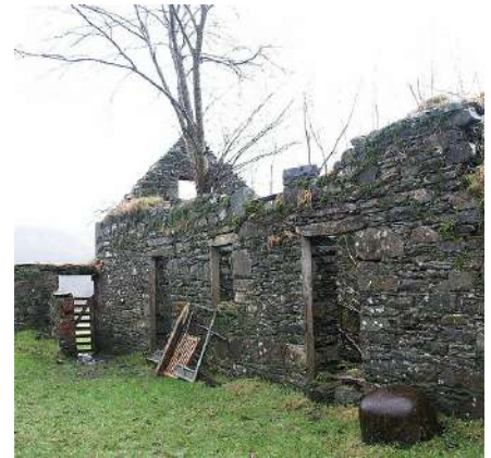
On some renovation projects, it is only the walls which are being renovated; the rest is really all new
