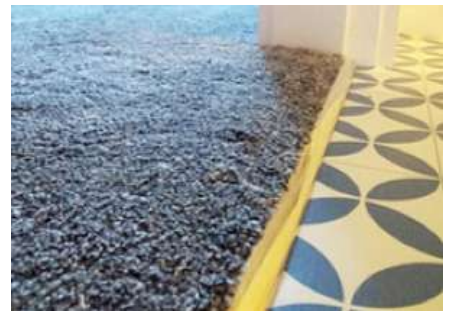
Many planned 10mm clear undercuts are compromised by later carpet installations
