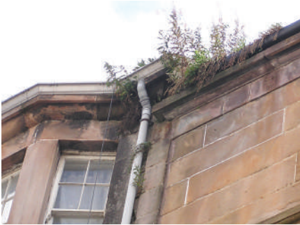
One of the most common problems is of blocked gutters and downpipes
