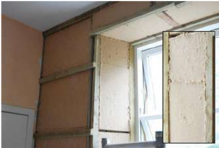
Top image: rigid insulation board installed fairly neatly, but there are still gaps through which heat, air and moisture will flow.
