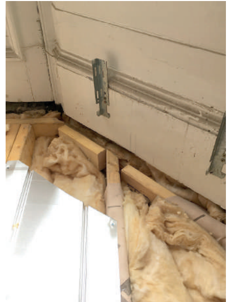
Insulation doesn't neatly fill the cavity, the membrane does not continue across the floor, nor is it sealed to the surrounding walls. This will lead to a drop in performance around the floor edges similar to that shown in the images and diagram on the previous page.
