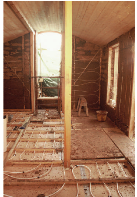
Underfloor and wall heating pipes installed on a small building in the Scottish Borders. Location of the pipes and the use of low level radiant heating pick up on both of the sections on human thermal sensitivity.
