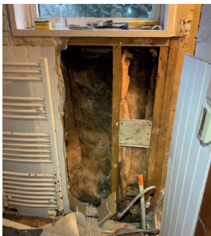
The insulation within timber frames is often far from adequate and so it is usually worth removing finishes to inspect before adding or adjusting insulation. This one shows not only that the insulation does not fill the cavity, but that inadequate vapour control has led to mould within the frame itself. If following the detail on the next page, this mineral wool should be removed, the frame dried out and new insulation installed with robust vapour control.
