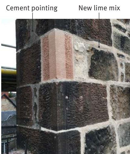
Cement pointing (still visible to the left) has been removed from the face of this chimney stack and replaced with a lime mix. In addition, a damaged stone has been replaced with a matching natural stone indent. In common with good conservation practice, the new stone matches the colour of the original, but the older stones have been heavily discoloured over time.
