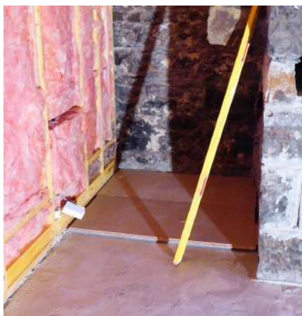
Aerogel blanket bonded to chipboard used as a thin, but high performance insulation over a solid floor. These boards would need to be taped to each other and to the surrounding walls to reduce associated air leakage.
