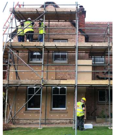
In this project, wood fibre EWI is being installed over a solid brick property © Natural Building Technologies
