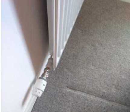
Thermostatic radiator valves, or TRVs, allow each radiator to be individually controlled meaning different rooms can be kept at different temperatures to suit different requirements
