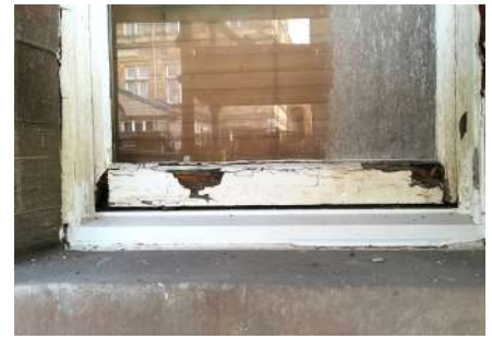
The rotten cill of this window has been removed and replaced with new, primed timber, while the lower rail and lower parts of the adjoining stiles of the window are due to be replaced. The paintwork will then need rubbed down and recoated, and a new sand mastic seal installed between the window and stonework.
