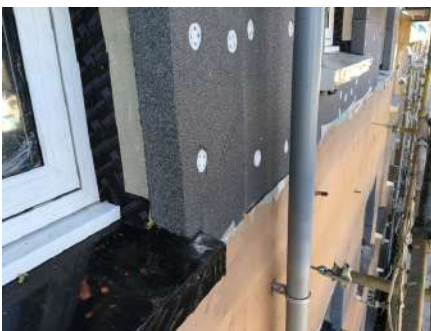
In the same project note airtightness tape (black) is affixed externally to prevent air getting in through the gap
