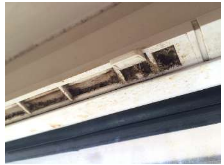
This kitchen trickle vent was completely blocked by debris mixed with grease
