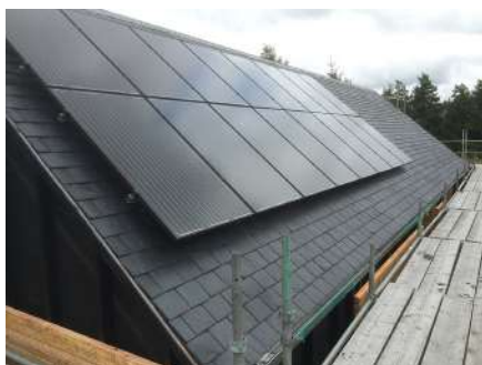
These PV panels are mounted on an existing slate roof
