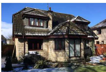
This timber frame house was built in the 80s but had a number of insulation gaps which needed to be resolved in order to reach the expected comfort levels
