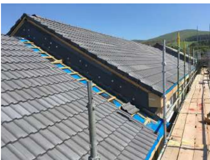
This image shows insulation applied to the upper levels of the gable. This area is often ignored but a small section of the upper flat has been insulated here.
