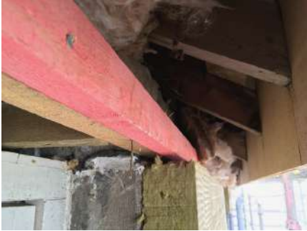
It is important that the roof insulation above meets the EWI below.
