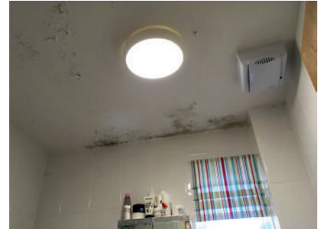
A scene that is familiar to thousands of households. The mould is due to a combination of excess moisture, cold surfaces and inadequate ventilation. It will impact on the health of the people using that room, and, over time, the condition of the building fabric.
