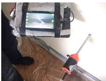
A borescope survey of a cavity wall showing the borescope inserted into the wall. The screen shows a tidy—and empty—cavity and a wall tie that is not straight.
