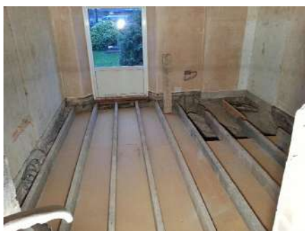
In this renovation, vapour permeable boards were used to contain the insulation, they were taped along all edges before the insulation was installed
